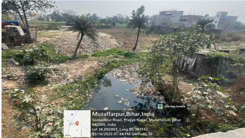
Drain outfall into Kadane River
